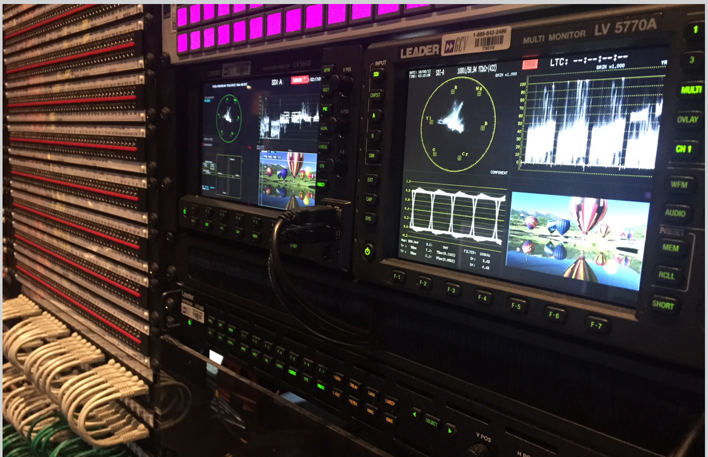
Courtesy Game Creek Video – Bravo truck installation of Leader LV5600 and LV5770A. Integration by Icon Broadcast
