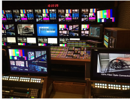
Interior of NEP's ND-1 truck, which relies on a 192 X 96, 9ME Grass Valley Kayenne production switcher.
