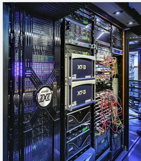
IP Router in SSCBS Mobile Unit.
