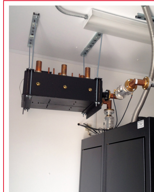
This hanging mask filter is connected to the transmitter output and the antenna transmission line. Note the probes on the filter input and output to monitor power and VSWR.
